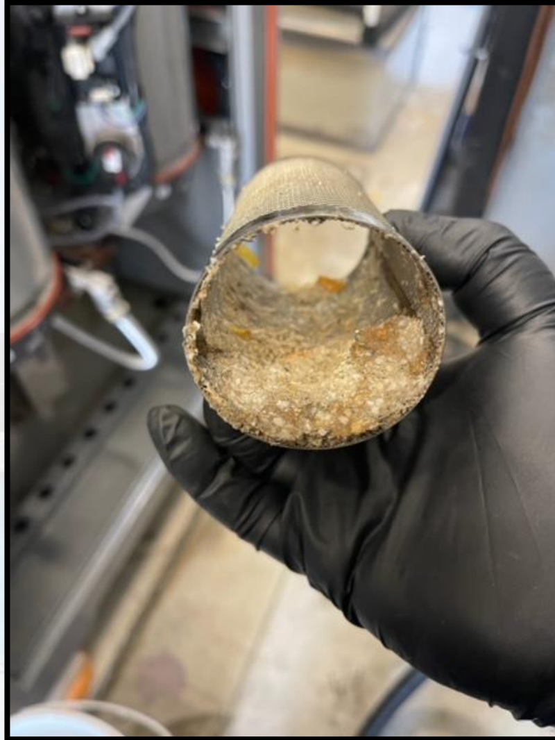
Hard limescale in the water heater's strainer
