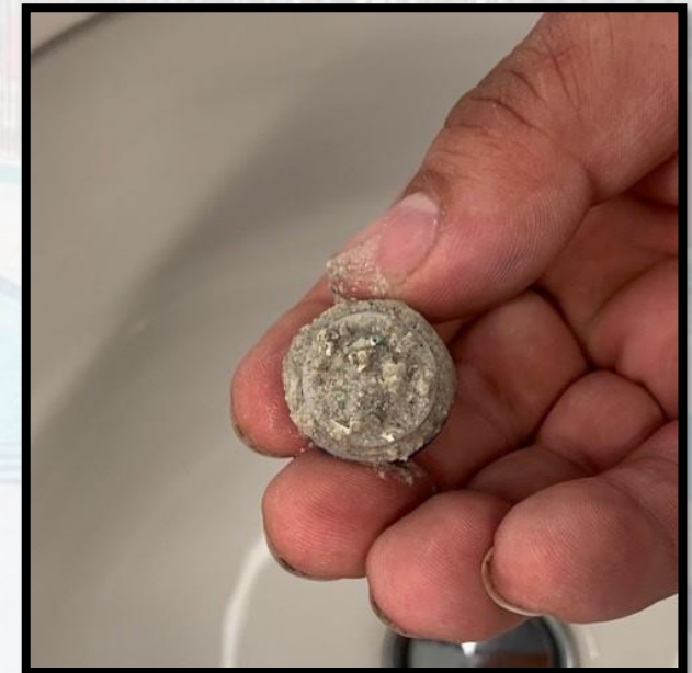
Plugged-up a faucet aerator
