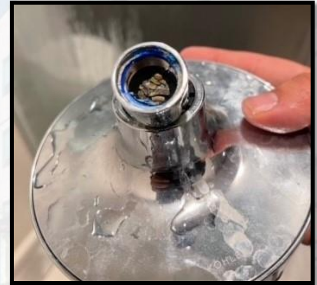
Limescale chunks in showerhead
