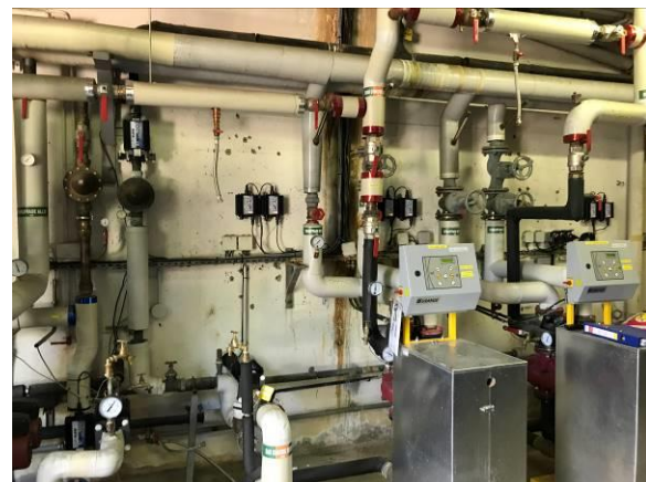
Main substation equipped
