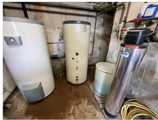
DHW tank Villa EXCELSIOR
