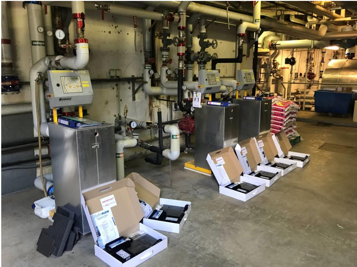
The 3 DHW production exchangers totalling 1450 kW of DHW production before installation
