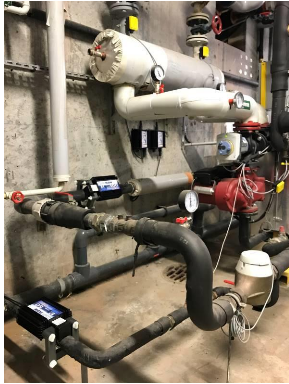
200kW Balneo exchanger
