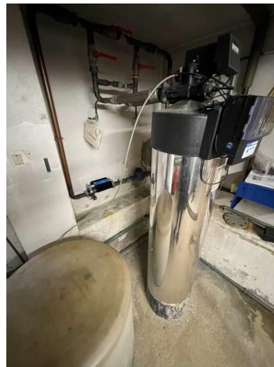
DHW tank Villa OLRy
